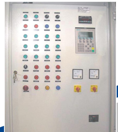
The Control Panel, containing an integral computer
