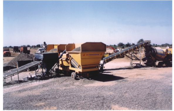
Plant working for (RMC) Ready Mix Set-up
